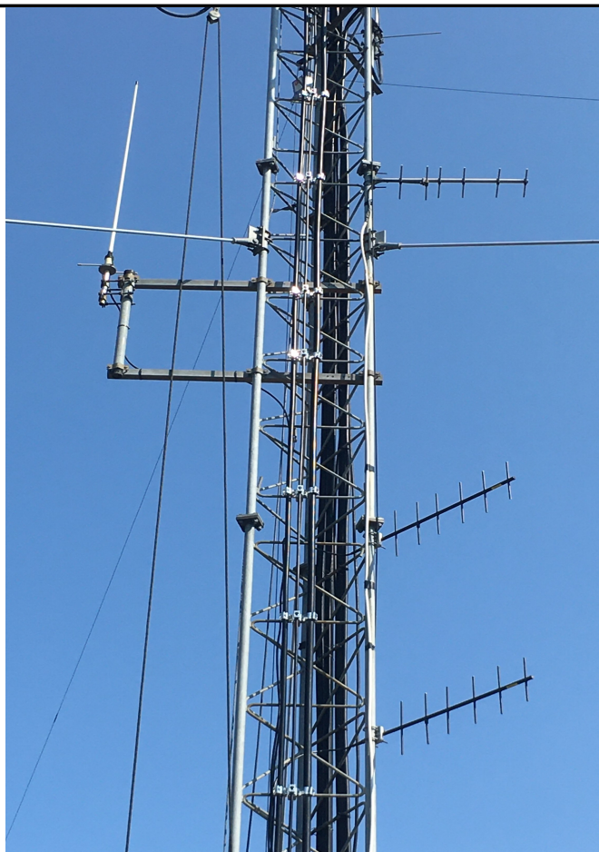
ANTENNAS TO LINK REPEATERS
