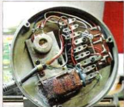
Figure A — This is why you should inspect any equipment that contains a battery. Fortunately, in this case, the corrosion had not yet gotten to the electronics in the stand.
