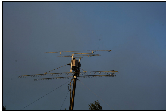
This photograph shows the microwave stack - 900Mhz - 10Ghz
