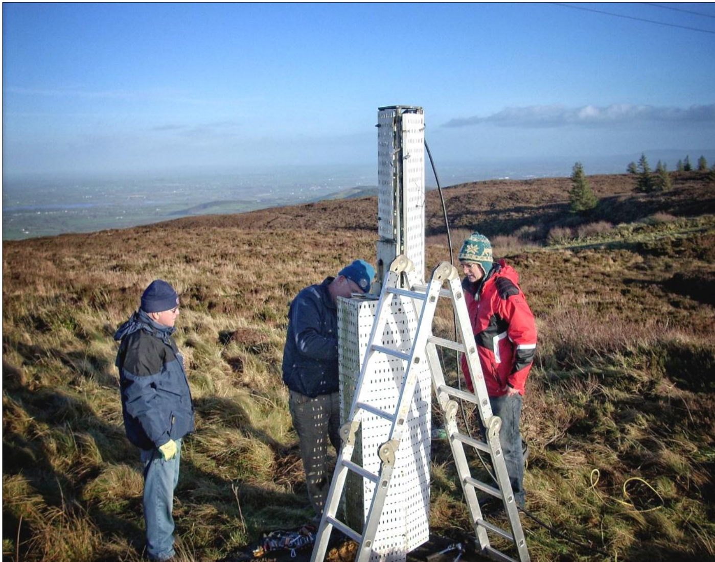
Limerick Radio Club - Harry EI3KL, John EI5HGB, and John EI1694 repair the 2m Repeater - Photo EI7ALB
