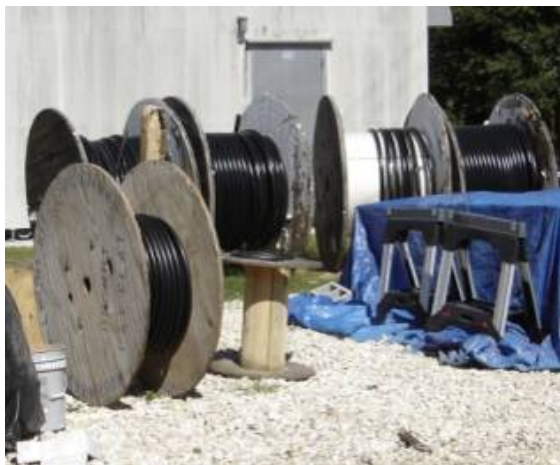
Heliac storage area
