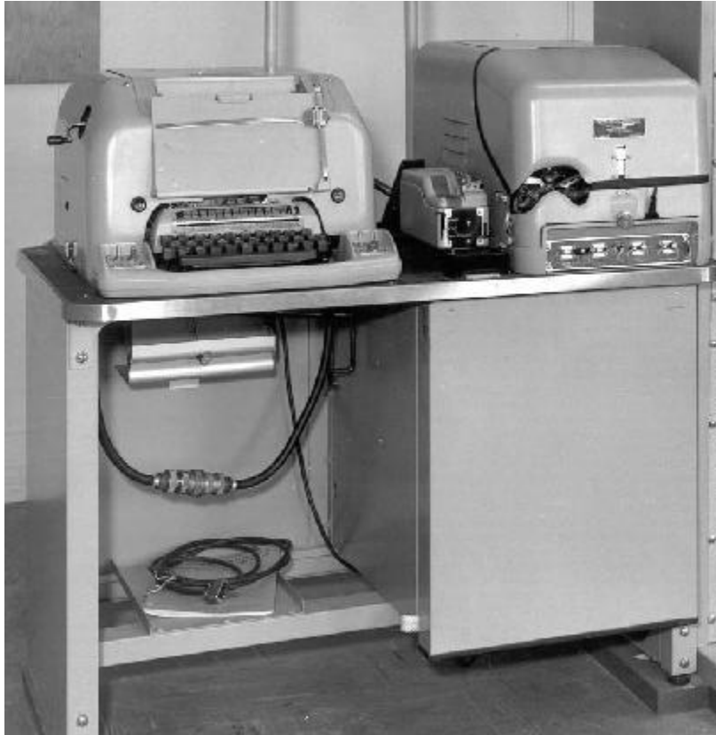
Modified AN/FGC-25 in AUTODIN Terminal Installation
