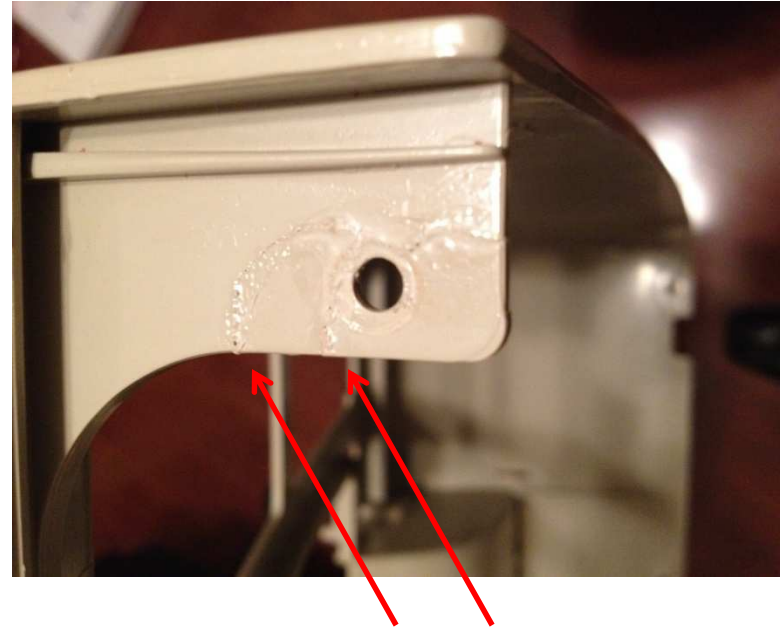
Front View after solvent weld. NOTE: Two full breaks in plastic.
