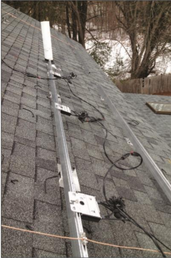
Figure 6 — The chokes from Figure 2, as well as the twisted wire transmission cables can be seen between two of the aluminum support rails before solar panels were installed.
