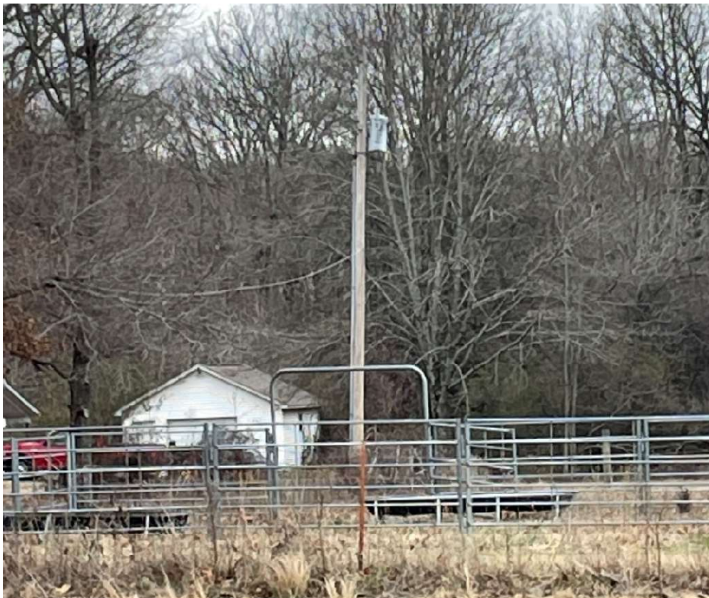
Figure 4 – Residence Service Pole 498 63 6 at 2924 Highway 157
